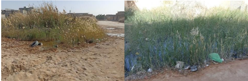
Figure 6: Groundwater surfacing in Al-Farjan (Right) and 7th of October (Left) neighborhoods, showing Pool Formation and associated Weed growth.
