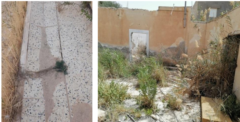
Figure 7: Ground Subsidence (Left) and Rising Dampness (Right), Resulting in the Abandonment of Several Residential Buildings.
