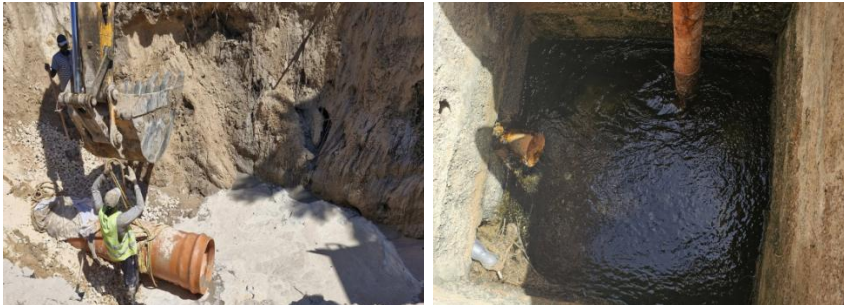
Figure 10: Dewatering well and Line in Zliten (Higher Technical Committee for Monitoring the Groundwater Overflow Phenomenon page, 2026).
